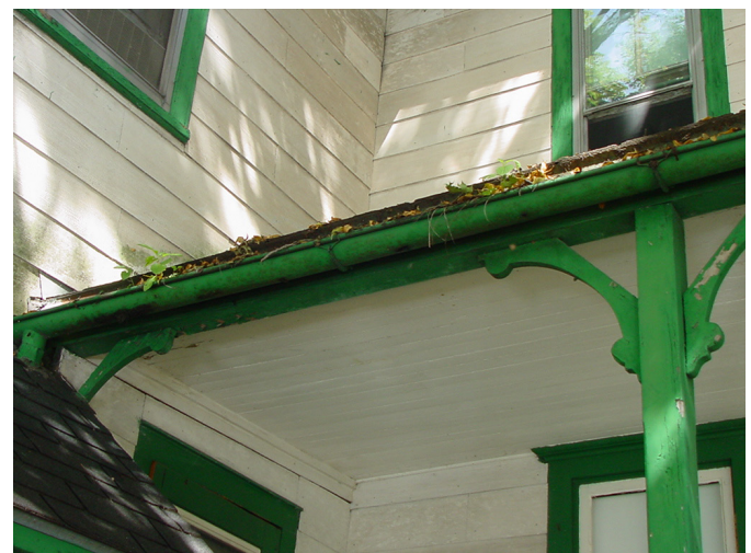
Gutters full of leaves and debris
