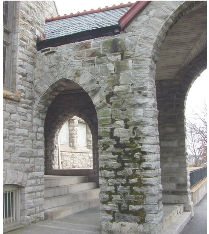
Damage caused by missing downspouts
