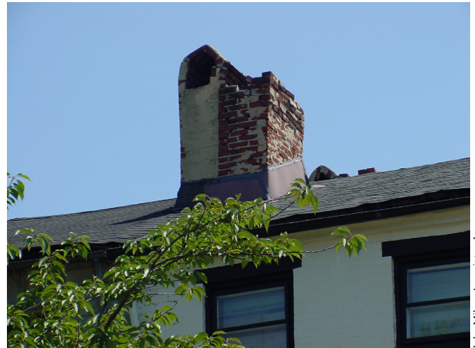
Example of chimney deterioration
